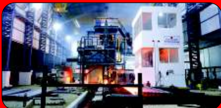
Continuous Casting Machine
